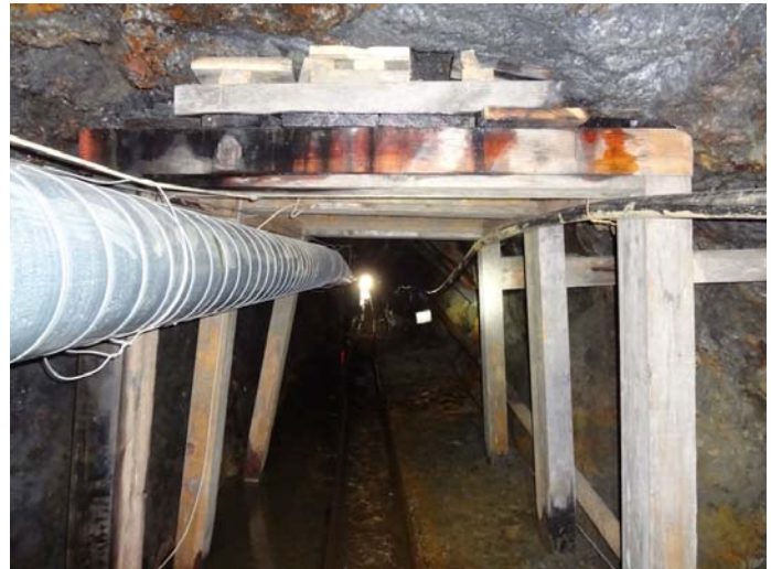
Rehabilitated Ruby Mine Tunnel (looking toward portal) Note New Timbers and Ventilation Duct Source: Analyst
